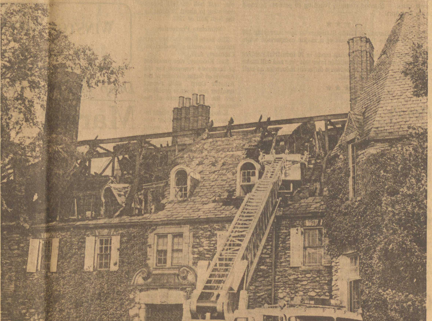
Photograph taken the day after the fire shows that little remains of the roof.
