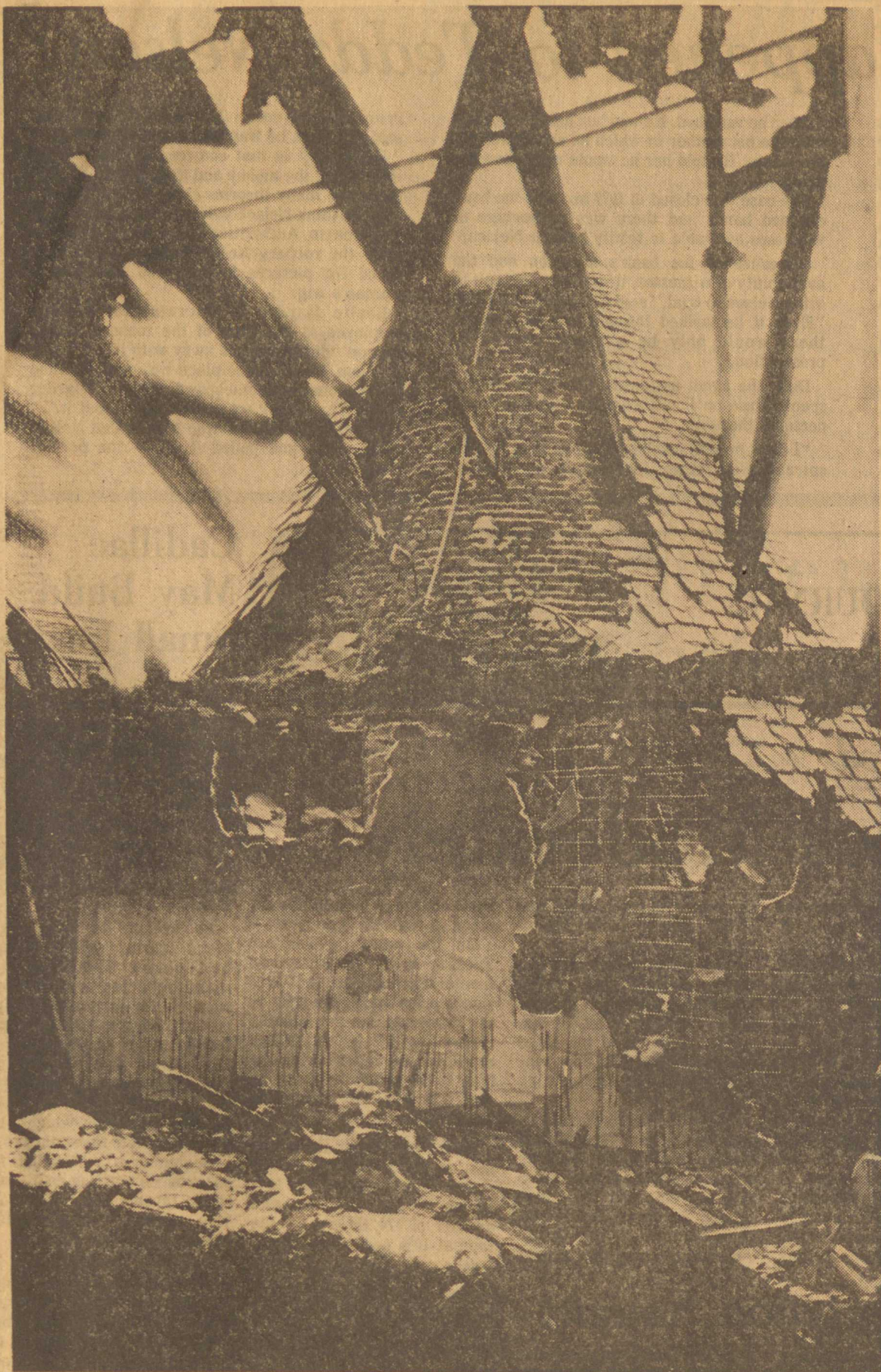
Graylyn turret still stands amid ashes and charred rubble on upper floor.
