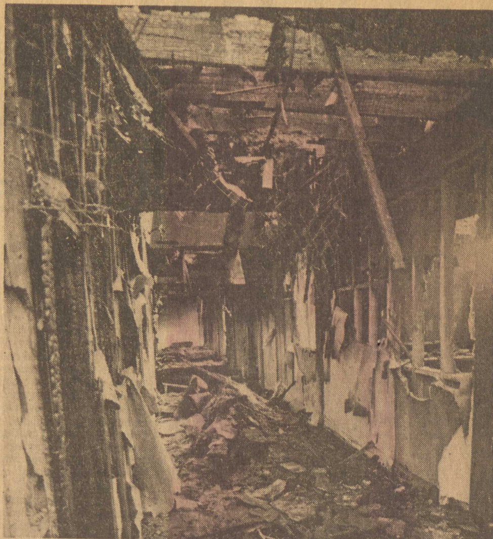
A hall on the third floor is a shambles.
