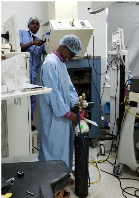
Figure 14: Suction blockage repair in Theatre Department
